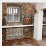
On damp masonry
