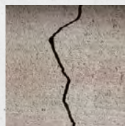
For dry cracks
