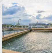
Collection and storage tanks
