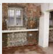
On damp masonry
