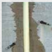
Forms foam in wet cracks
