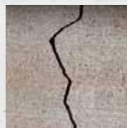
For dry cracks
