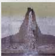
For water bearing cracks
